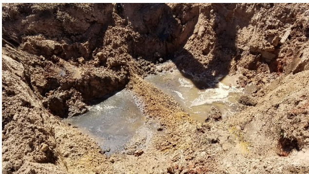
Photo #31: Tank Pit #2 : Perched Water in Pit
