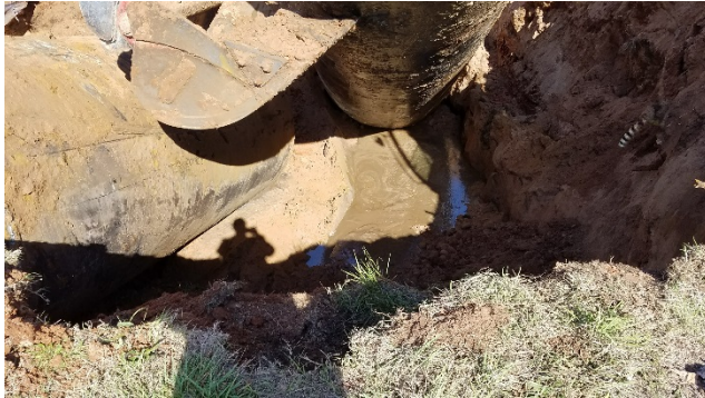
Photo #13: Underside of Tank # and Perched Water Below
