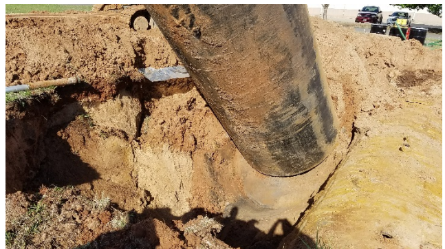
Photo #12: Underside of Tank #1 and Soil Below
