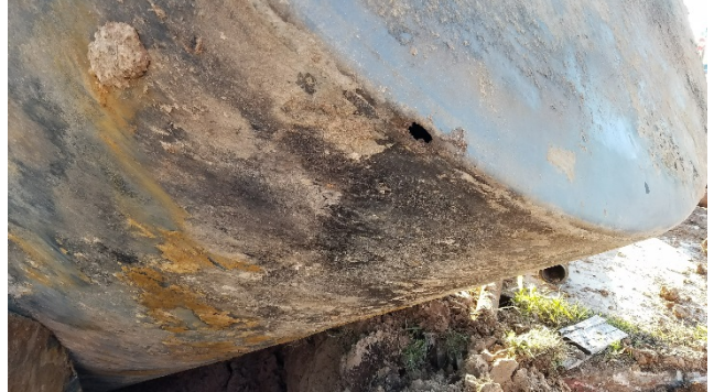
Photo #28: Corrosion Hole in Tank #4
