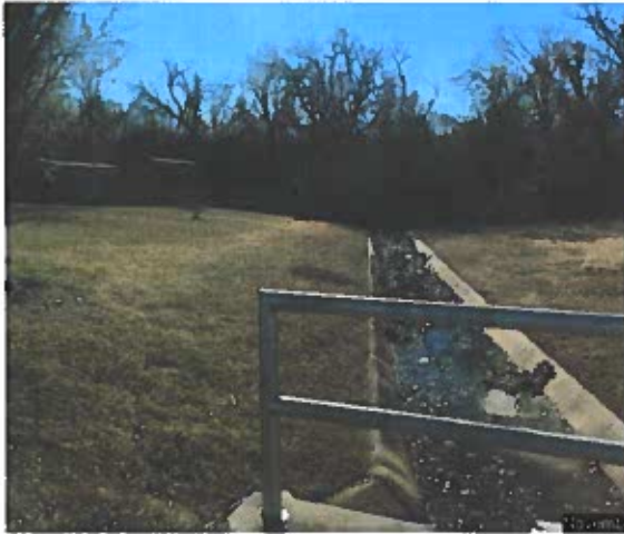
Looking south from Alicia Drive where all the drainage would cross under the road. The home owners of 10304 and 10316 Alicia Drive have fenced across the City's drainage easement. This fence will likely need to be removed to gain access for the grading work and future maintenance.
