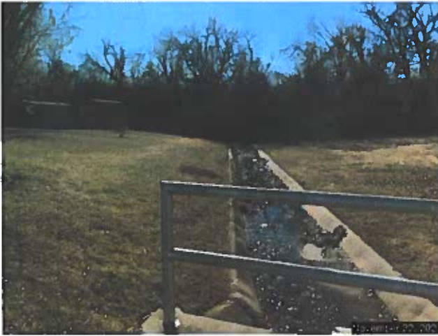
Looking south from Alicia Drive where all the drainage would cross under the road. The home owners of 10304 and 10316 Alicia Drive have fenced across the City's drainage easement. This fence will likely need to be removed to gain access for the grading work and future maintenance.
