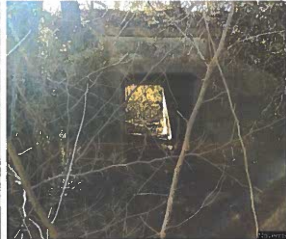
The box culvert under the railroad berm which would carry all the water from the south side of the berm. The box was constructed in 1931.
