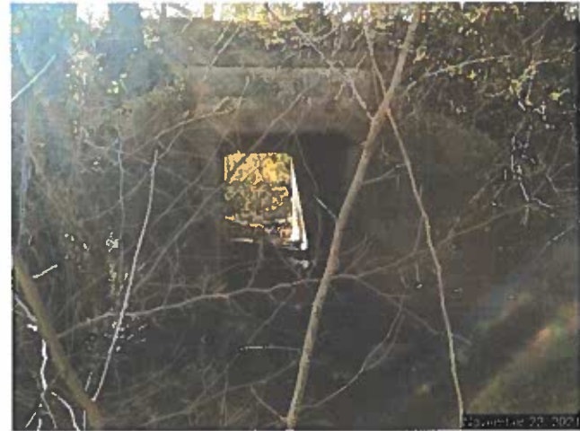
The box culvert under the railroad berm which would carry all the water from the south side of the berm. The box was constructed in 1931.
