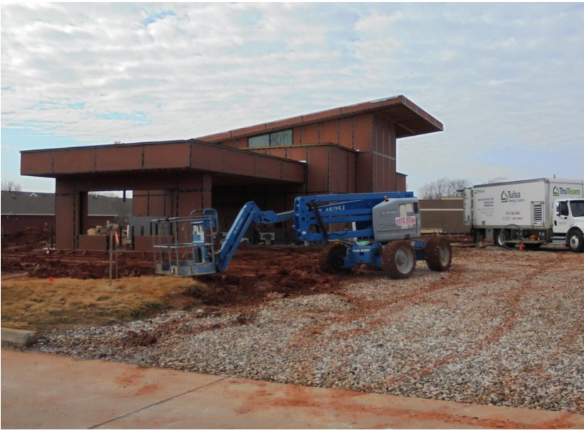
LEFT: U.S. Employees O.C. Credit Union is under construction at the SW corner of S Davidson Road and E Reno Avenue.
