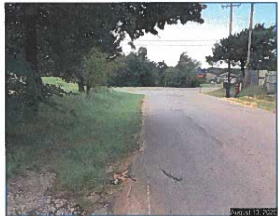
Looking west on SE 28 th Street. No curb and gutter or sidewalk. Note the poor condition of roadway surface.
