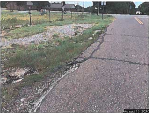
Looking west on SE 10 th Street. No Curb and Gutter or sidewalk. Note the poor condition of roadway surface.
