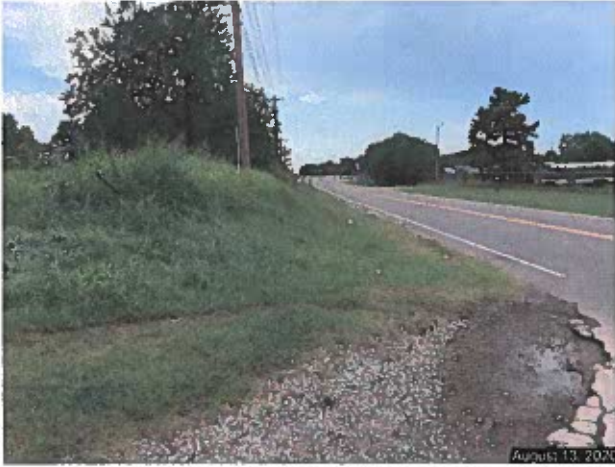
Looking south at corner of SE 28 th Street and Westminster Road. No Curb and Gutter or sidewalk. Note the poor condition of roadway surface.
