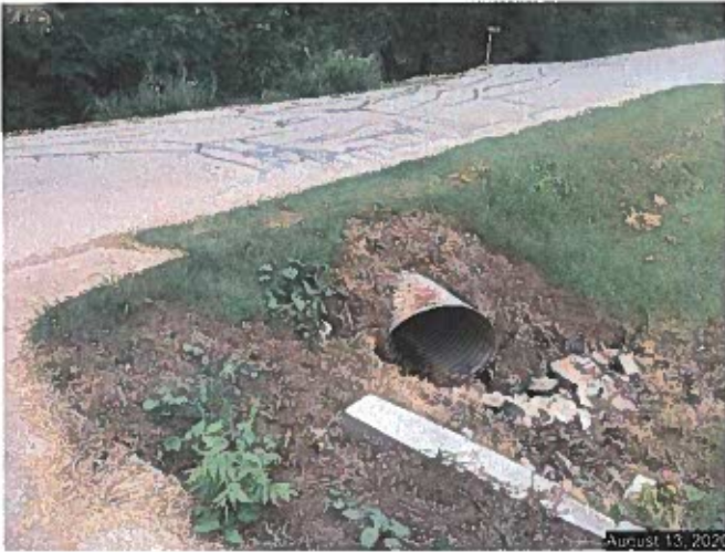
Crossdrain downstream where water flows under SE 28 th Street to the north northeast
