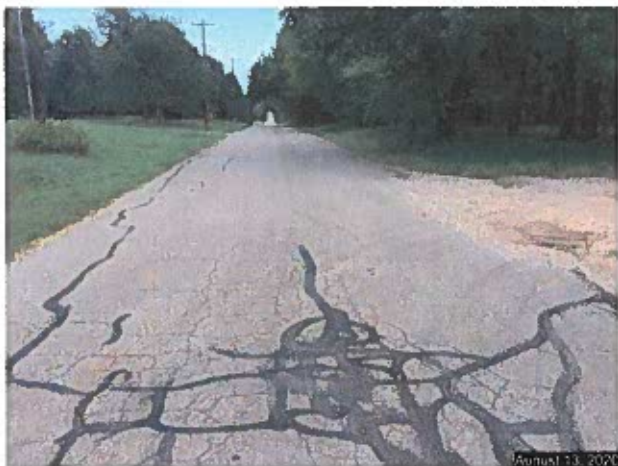
Looking east on SE 28 th Street. No Curb and Gutter or sidewalk. Note the poor condition of roadway surface.
