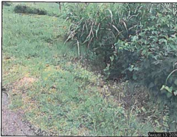
South side of SE 10 th Street, outflow of 24" cross drain opposite inlet.
