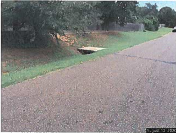
North side of SE 10 th Street, inlet catching water and taking it via 24" pipe to east side of property in question.
