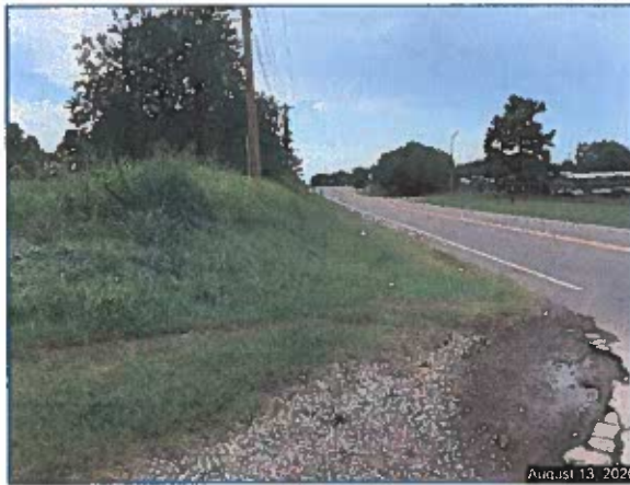
Looking south at corner of SE 28 th Street and Westminster Road. No curb and gutter or sidewalk. Note the poor condition of roadway surface.
