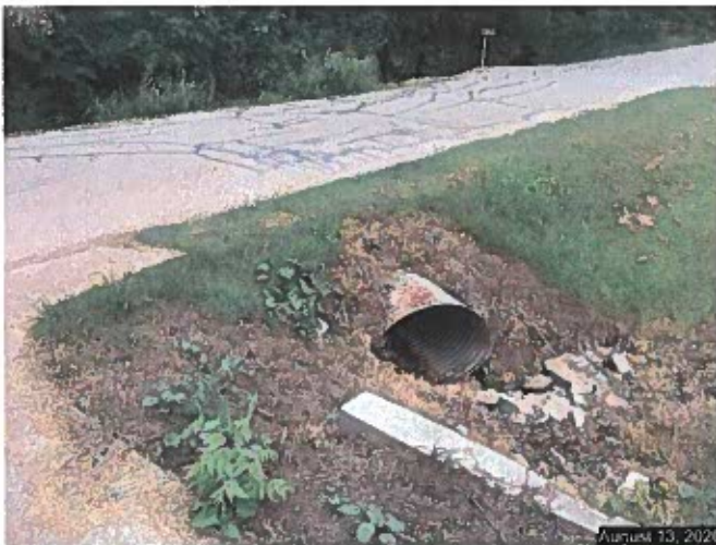
Crossdrain downstream where water flows under SE 28 th Street to the north northeast
