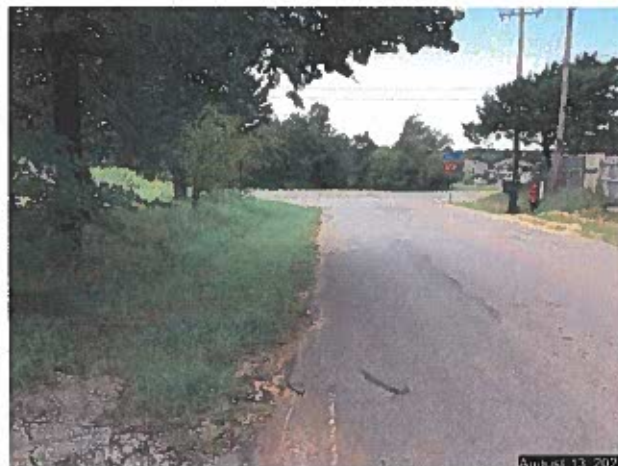
Looking west on SE 28 th Street. No Curb and Gutter or sidewalk. Note the poor condition of roadway surface.
