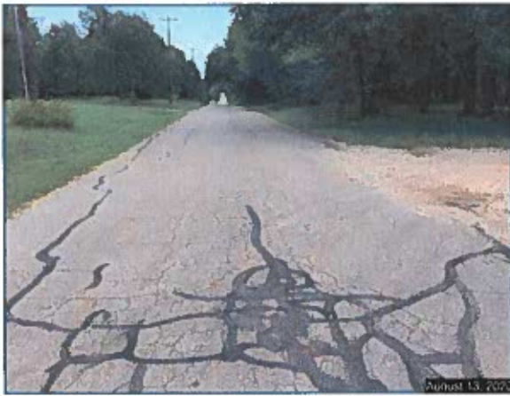
Looking east on SE 28 th Street. No curb and gutter or sidewalk. Note the poor condition of the roadway surface.
