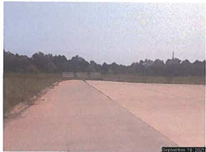
Looking south on America Avenue near the intersection of S.E. 20 th Street. Barricades set for future extension (not on this phase).
