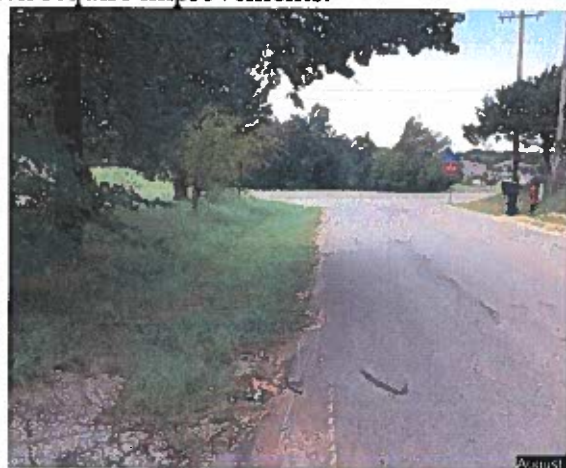
Looking west on SE 28 th Street. No Curb and Gutter or sidewalk. Note the poor condition of roadway surface.
