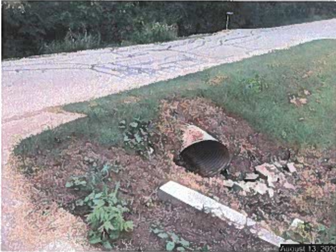
Crossdrain downstream where water flows under SE 28 th Street to the north northeast
