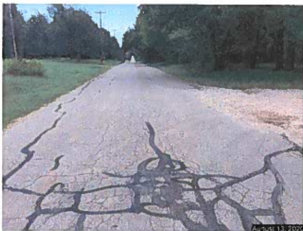
Looking east on SE 28 th Street. No Curb and Gutter or sidewalk. Note the poor condition of roadway surface.
