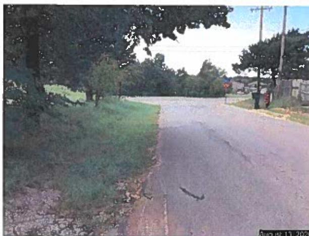
Looking west on SE 28 th Street. No Curb and Gutter or sidewalk. Note the poor condition of roadway surface.
