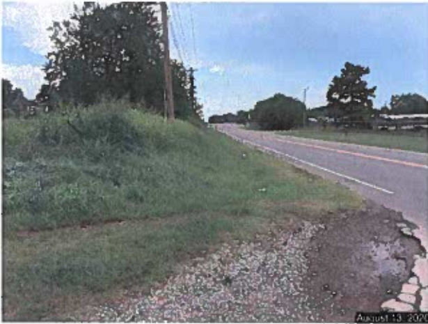
Looking south at corner of SE 28 th Street and Westminster Road. No Curb and Gutter or sidewalk. Note the poor condition of roadway surface.
