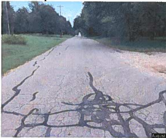
Looking east on SE 28 th Street. No Curb and Gutter or sidewalk. Note the poor condition of roadway surface.
