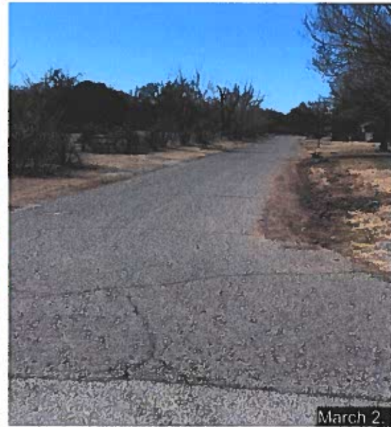
Looking west from intersection of NE 5 th Street and Oakview Drive along NE 5 th Street showing substandard street. Subject plat is on the south side (left in picture)
