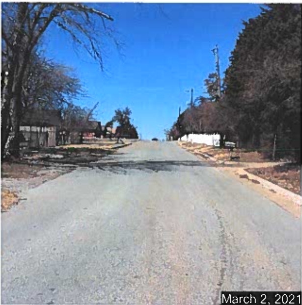
Looking north from intersection of NE 5 th Street and Oakview Drive along Oakview Drive showing substandard street but curb and gutter existing along east side
